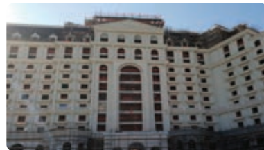
Vendome Mall, Lusail, Qatar All Inverter VRF Systems – 183 HP
