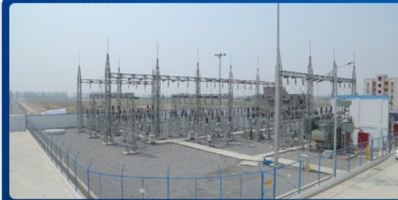
Tata Power Delhi Distribution
